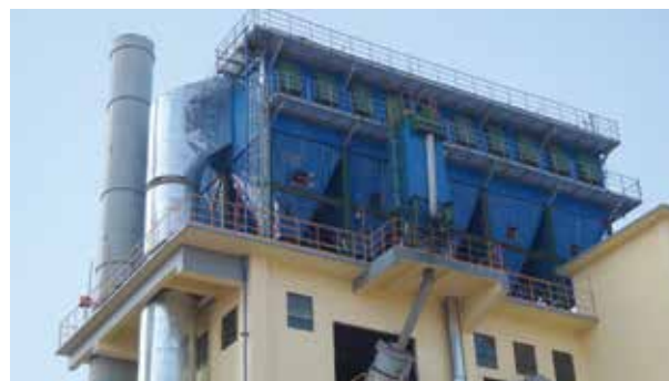
Bag filter for coal mill of Vietnam Xining Cement Plant
