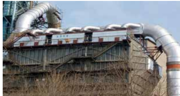
Conversion of high dust-laden kiln ESP to BF(4000t/d) for DOCC -The typical conversion case of high dust-laden kiln ESP to BF (16 days of kiln shutdown).
