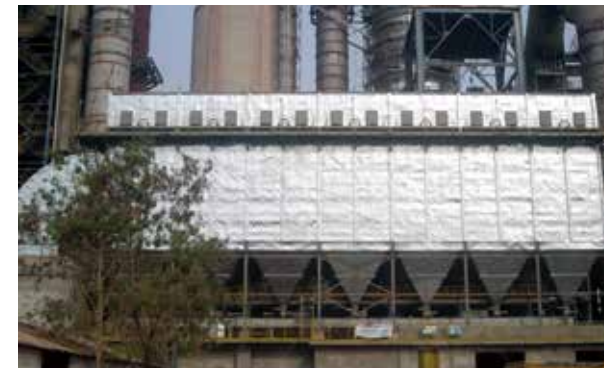
Bag filter for kiln of Lafarge India Sonadih Cement Plant ( 5000 t/d )
