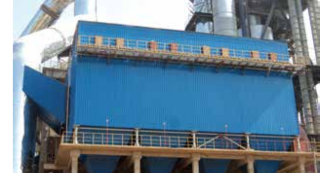
Bag filter for kiln of Guangdong Youkeng Building Material Co. ,Ltd. ( 5000 t/d )
