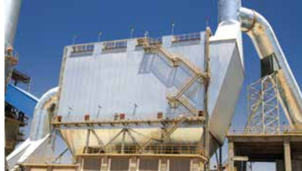
Electrostatic precipitator for cooler of Egypt Nahada Cement Plant( 5000 t/d )
