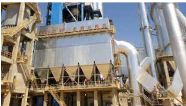
Bag filter for bypass of Egypt Nahada Cement Plant( 5000 t/d )
