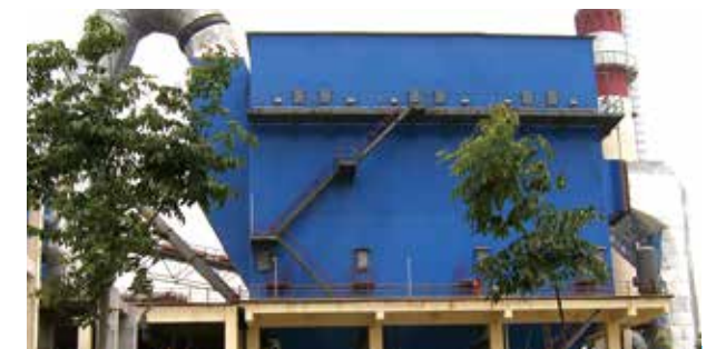
Conversion of cooler ESP to BF (5000t/d) for Jiaomei Group QianYe Cement Plant-The first conversion case of cooler ESP to BF in China.
