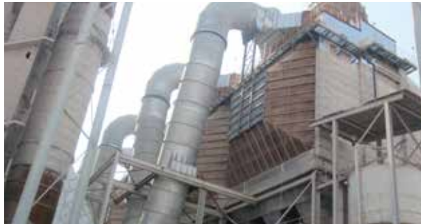
Conversion of cement mill ESP to BF (5000 t/d) for Saudi Arabia SCC Cement Plant
