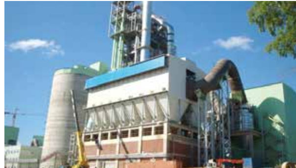
Joint bag filter for kiln and cooler of Heidelberg Russia Tula Cement Plant( 5000 t/d )
