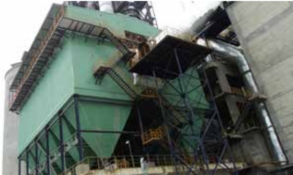
Bag filter for kiln of Lafarge Sancha Cement Plant ( 5000 t/d )
