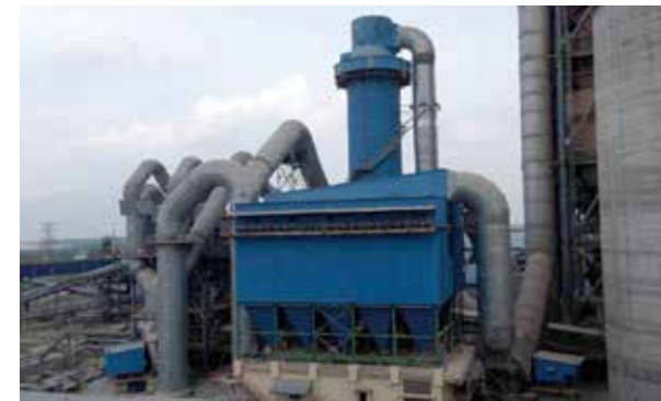
Bag filter for kiln of Malaysia Hume Line 2 Cement Plant (5000 t/d)
