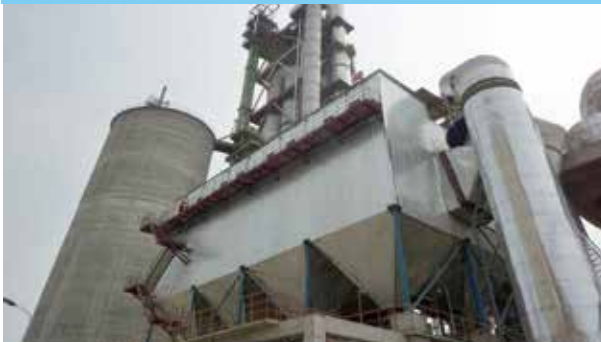
Bag filter for kiln of Sinoma Hanjiang Cement Plant (2500 t/d)
