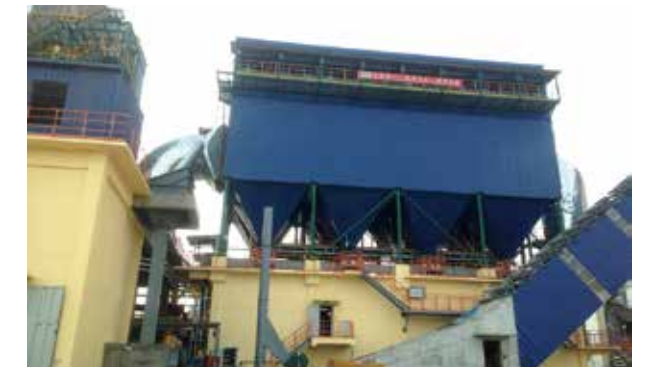
Bag filter for cooler of Malaysia Hume Line 2 Cement Plant (5000 t/d)
