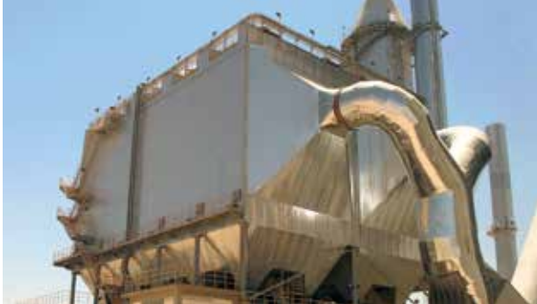
Electrostatic precipitator for kiln of Egypt Nahada Cement Plant( 5000 t/d )
