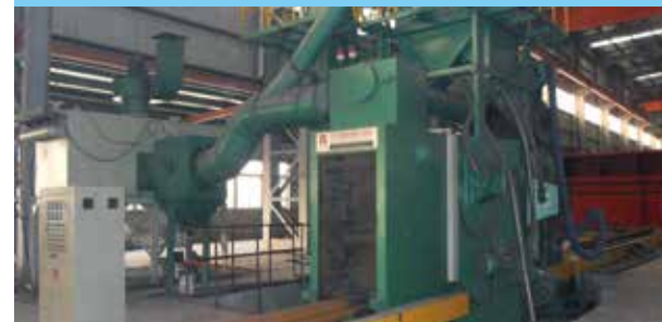
Steel structure pretreatment equipment
