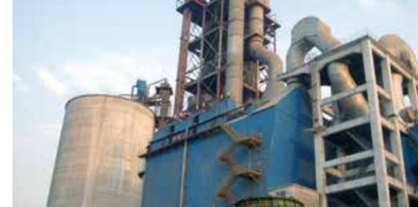
Conversion of high dust-laden kiln ESP to hybrid dust collector (5000t/d) for Tianrui Group Ruzhou Cement Plant-The first conversion case of high dust-laden kiln ESP to hybrid dust collector in China (13.5 days of kiln shutdown).
