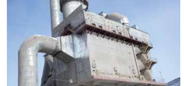
Conversion of kiln ESP to BF (2000t/d) for Halaer Mengxi Cement Plant- especially designed for extreme cold area.
