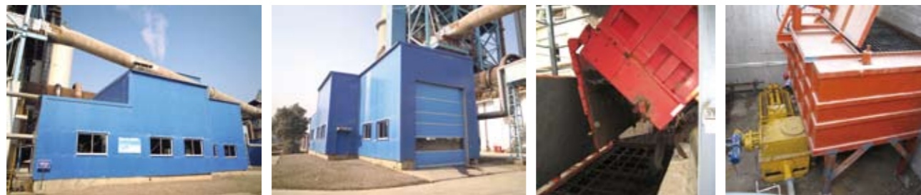
污泥接收及储存系统 Sludge receiving and storage system 全封闭的污泥接收单元 Fully sludge sealed unit 污泥运输车卸车 Sludge carrier vehicle unloading 污泥接收仓及输送泵 sludge receiving bin & delivery pump
