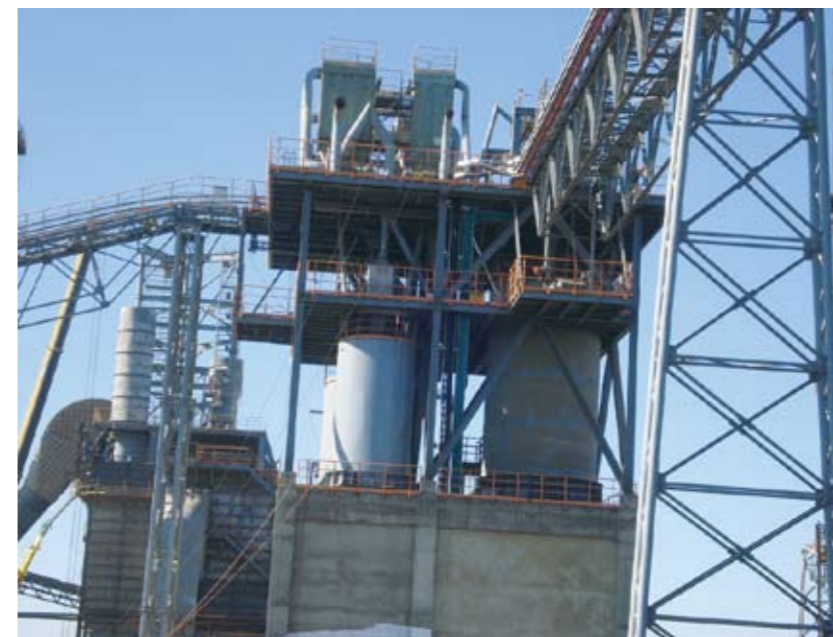
◀ 332原料调配车间设备安装收尾 332raw material blending workshop equipment installation ending
